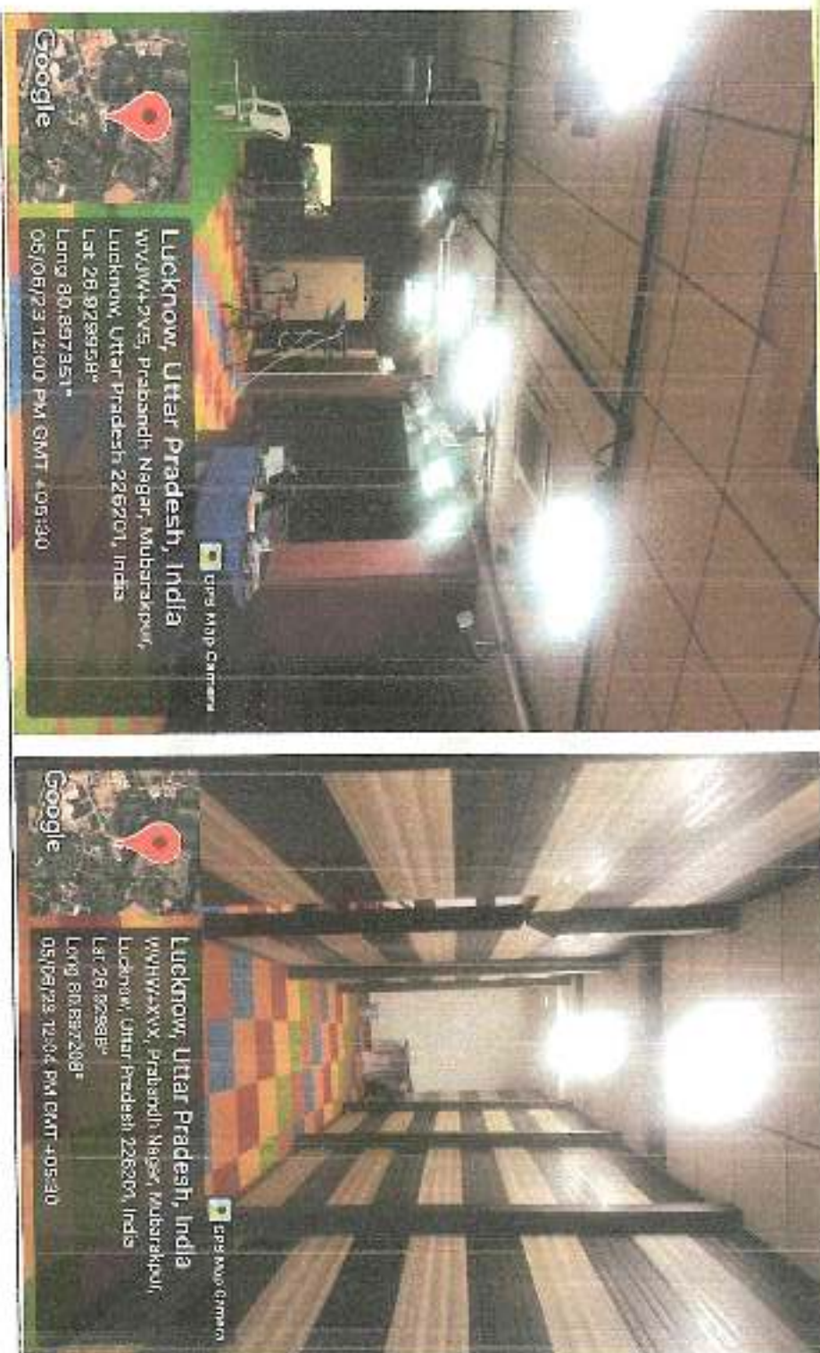
Indoor lighting fixtures at KMCIU
