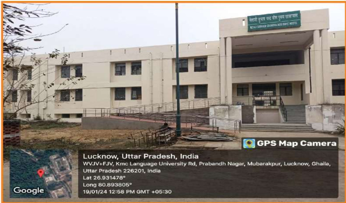
The installation of ramp-railings in Netaji Subhash Chandra Bose Boys Hostel for enhancing accessibility, ensuring that individuals with disabilities can navigate with ease and independence.
