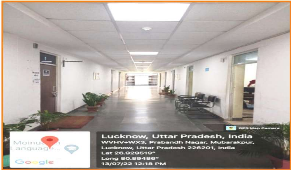
LED Panels in the Corridors of Academic Building
